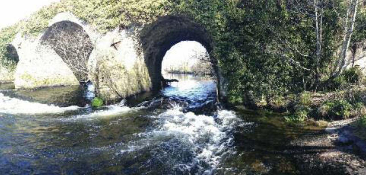
Ballyhilty Bridge spanning over the River Ilen. Image courtesy of 'StreamScapes Images/Jessica Mason'.
