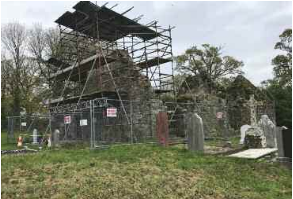
Church from south west, the west gable of nave undergoing conservations works.
