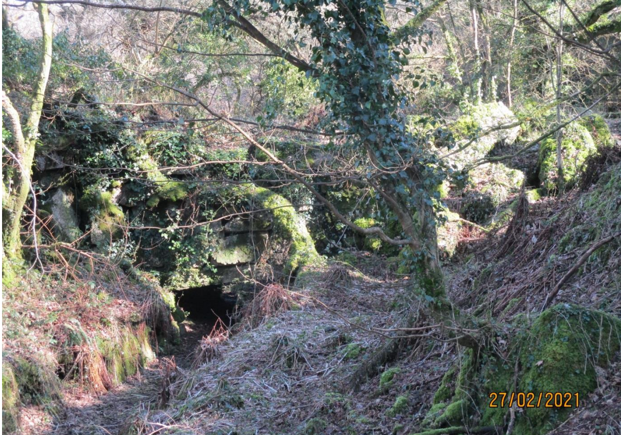
This finger dump 'bridges' the (now dry) Carmears leat so the quarry and leat could co-exist.
