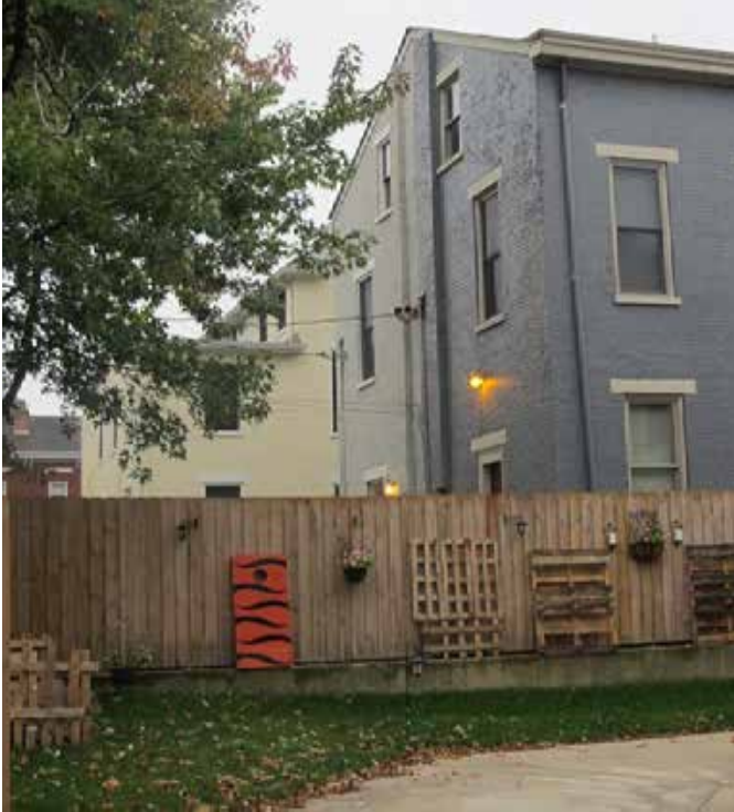
Whenever possible have electric, cable and other utility lines enter the building from the rear or ally
