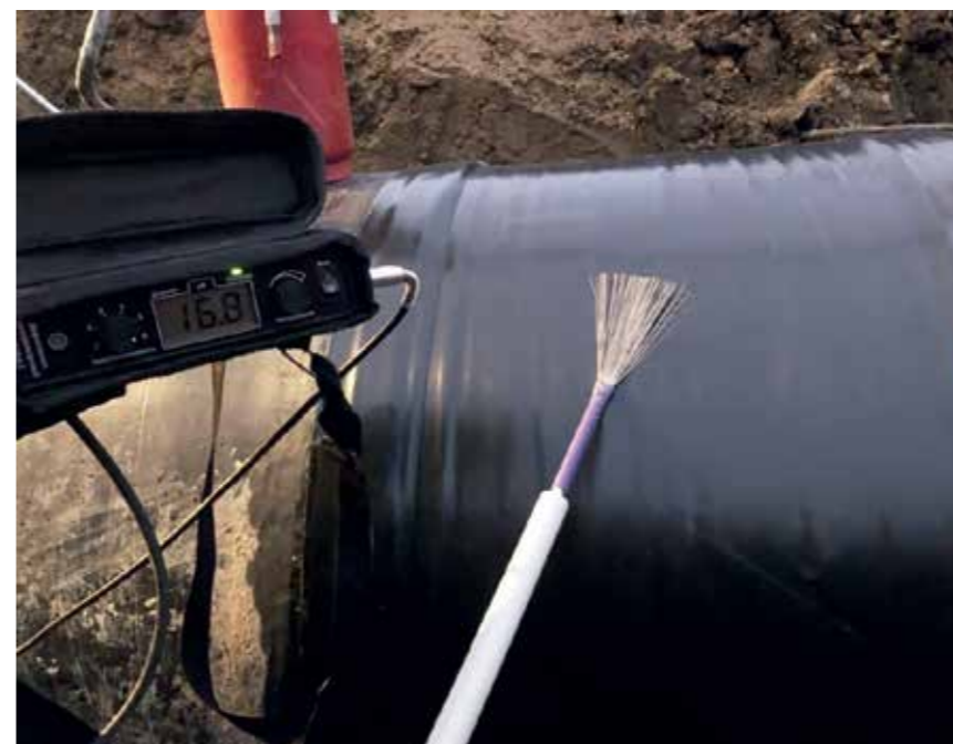
CHECKING THE QUALITY OF THE INSULATING COATING AT KM 1216 OF THE TENGIZ – NOVOROSIYSK OIL PIPELINE
