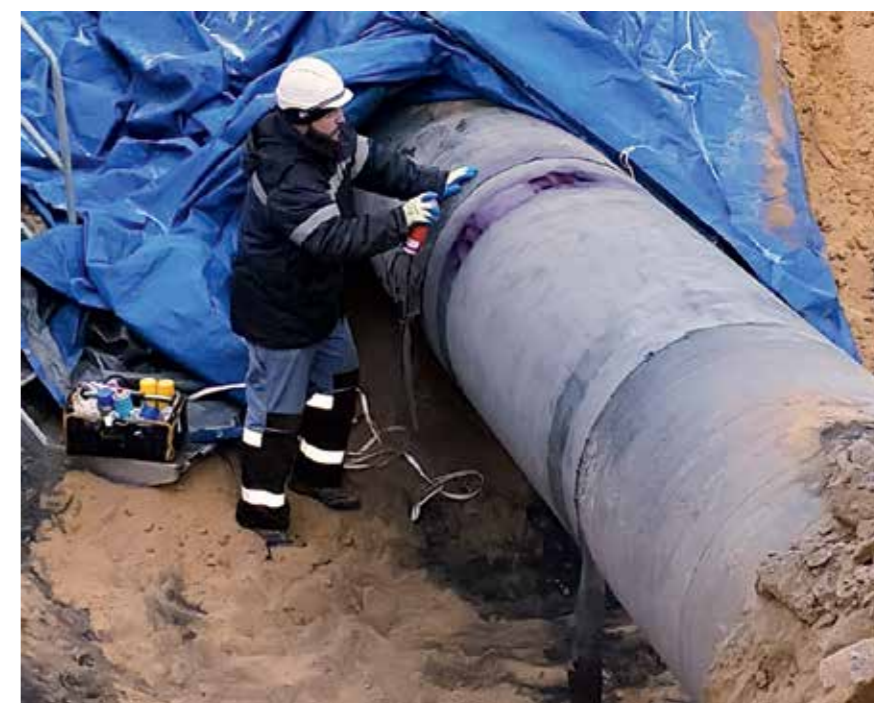
CAPILLARY CONTROL OF THE BASE METAL AT THE WELDING POINTS OF THE CIRCUMFERENTIAL JOINTS OF THE REPAIR STRUCTURE P2
