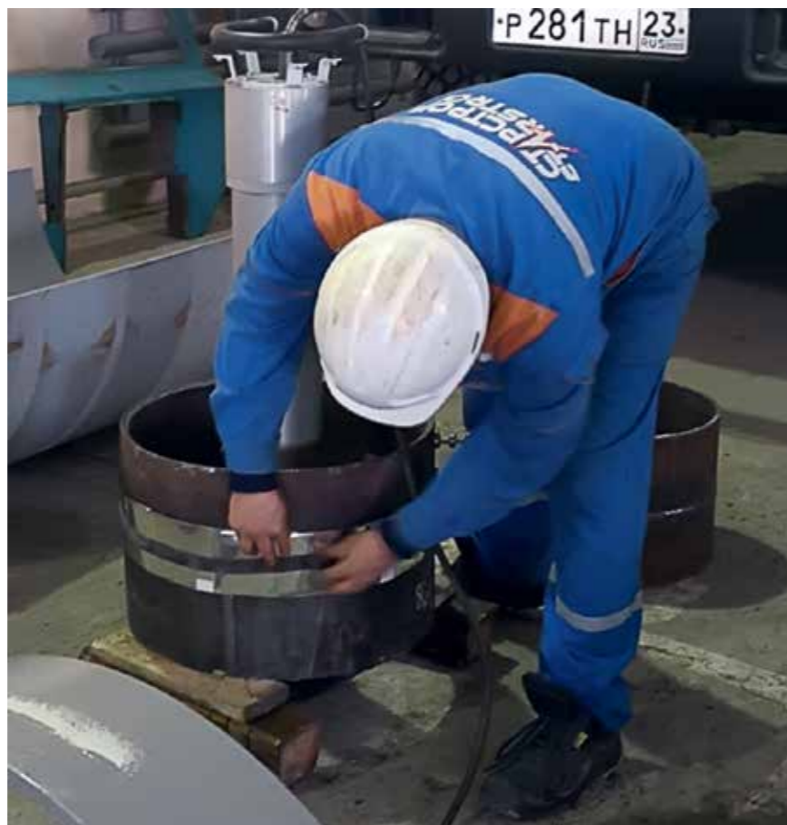
RADIOGRAPHIC INSPECTION OF A WELDED JOINT ON THE BASIS OF KROPOTKIN ERC
