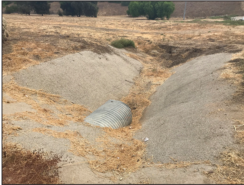
Photo 1 – View to the east illustrating the concrete swale (Swale 1) and culvert that ties into Swale 2. Overland sheet flow is collected in the swale and conveyed west through the culvert toward Swale 2 and Conejo Creek.
