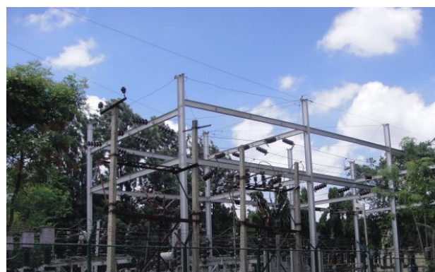
Figure 1: BESCOM switchyard in Cooke Town
