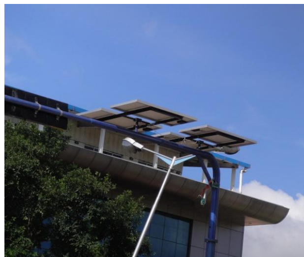
Figure 19: Solar PV powered traffic signals have become a common sight – Signal at J. P. Nagar
