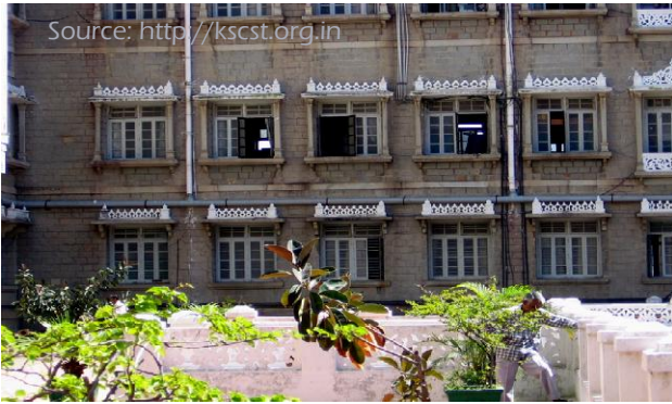
Figure 20: Rainwater collection pipes at Vidhana Soudha
