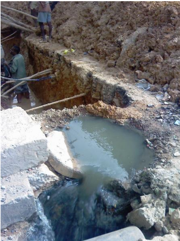
Figure 8: Overflowing manhole contaminating wells in the neighbourhood, Shivaji Nagar
