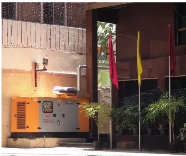
Figure 12: DG sets are becoming the norm – A hotel in central Bangalore
