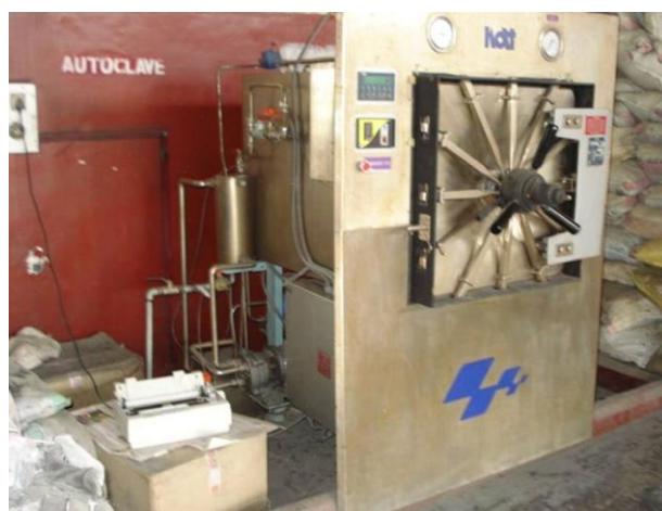
Figure 9: Autoclave for disinfection
