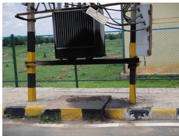
Figure 10: Oil leaking out of a transformer at Madivala tank bed
