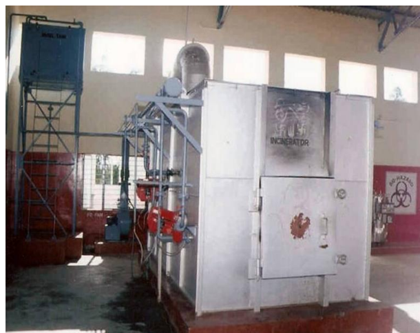
Figure 8: Dual chamber incineration facility
