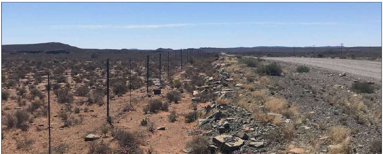
Figure 4.12: Contextual Images indicating the disturbed road surface
