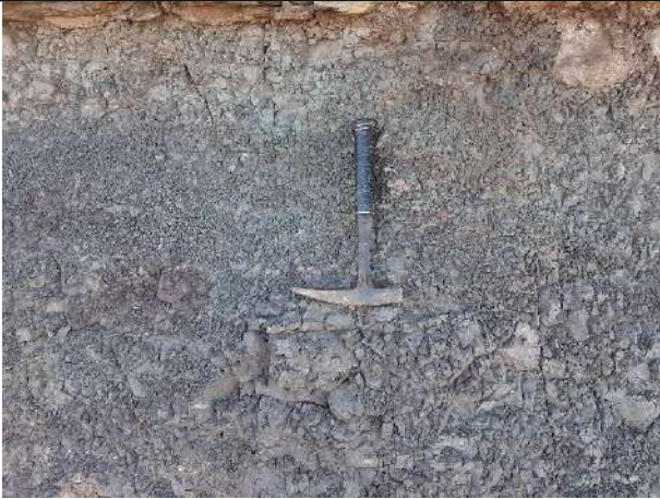
Figure 18 Highly fractured mudstones
