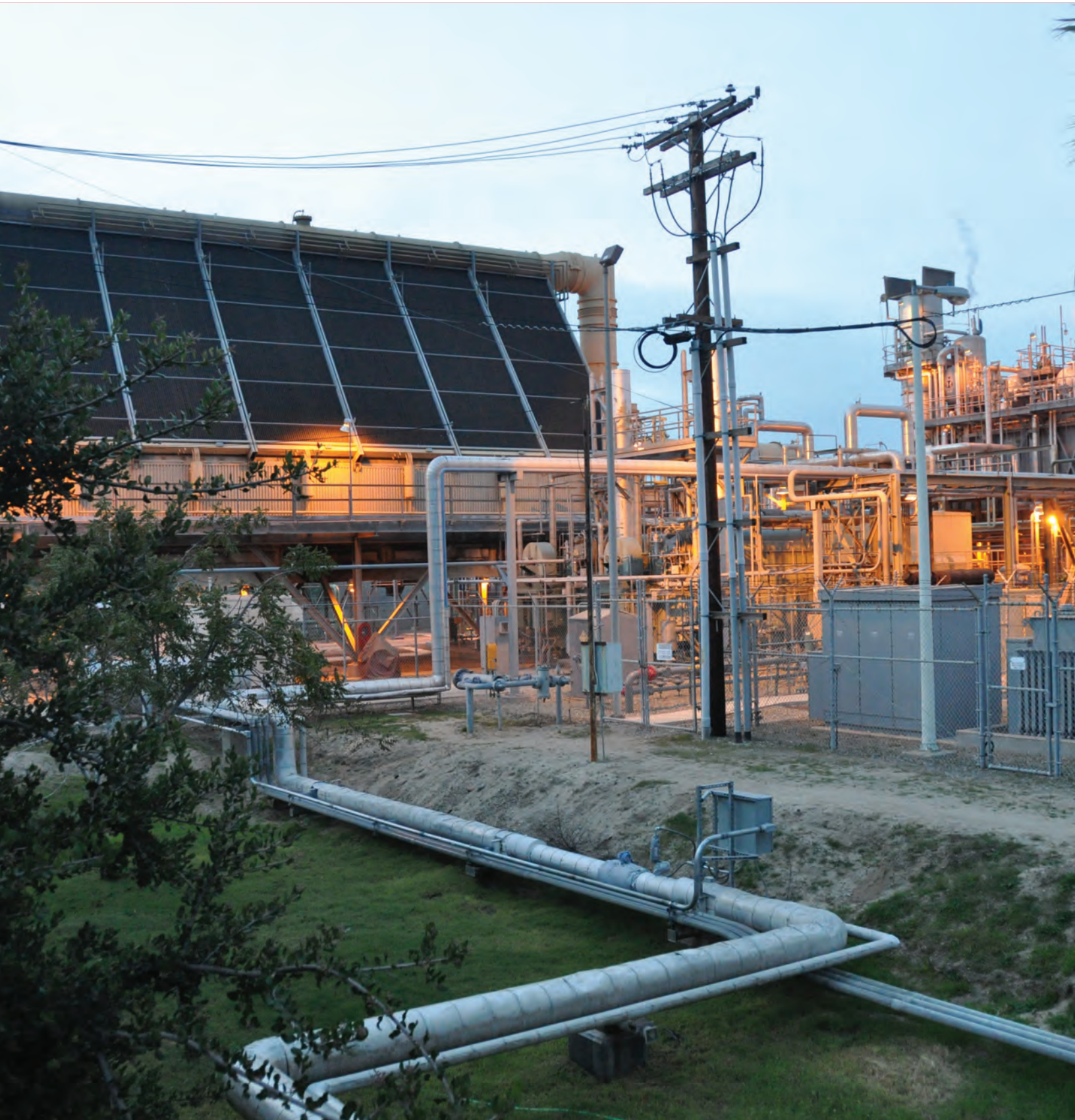
Co-Gen Plant on West Campus
