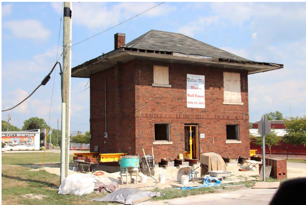
The Union City Interlocking Tower after being placed on its new foundation in Artisan Crossing Park.
