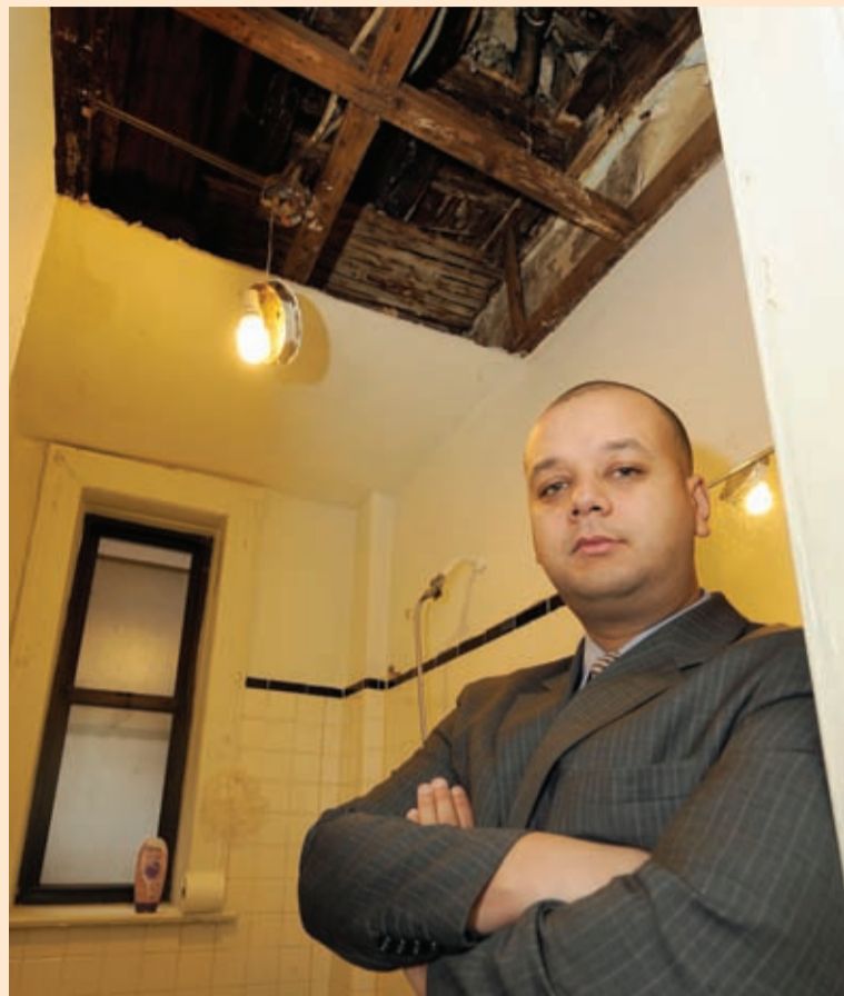
Attorney Pedro Rivera helped win compensation for tenants of unrepaired apartments including this one with a collapsed ceiling.
