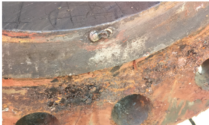
Figure 2. Bolted flange failure due to an AC fault on an unprotected joint
