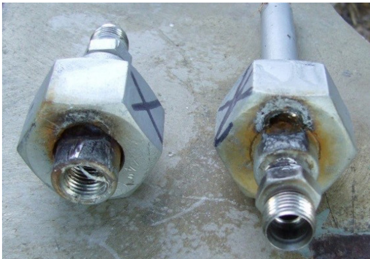
Figure 3. Rupture of a dielectric union resulting from an AC fault
