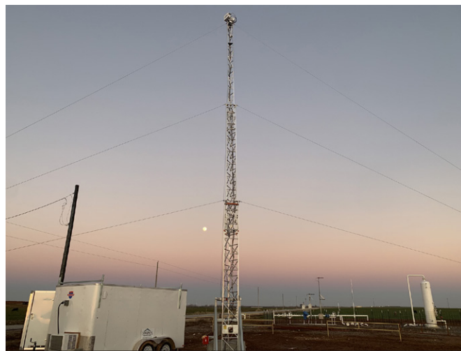
LongPath dual frequency comb emissions detection system installed in an oil and gas production field in Oklahoma. This system is continuously monitoring 20 complex multi-well facilities over a 17.5 square mile region.
