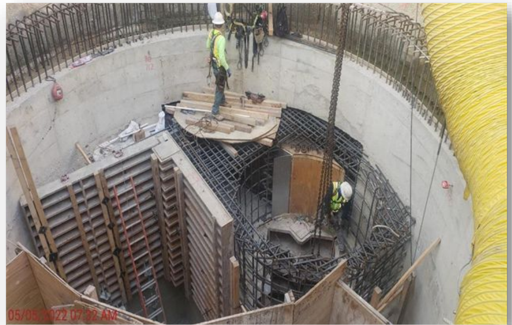
Drop Shaft Internals
