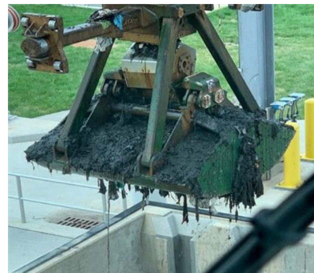
Trash, Debris and Solids Removal from Screening Shaft at Tunnel Dewatering Pumping Station
