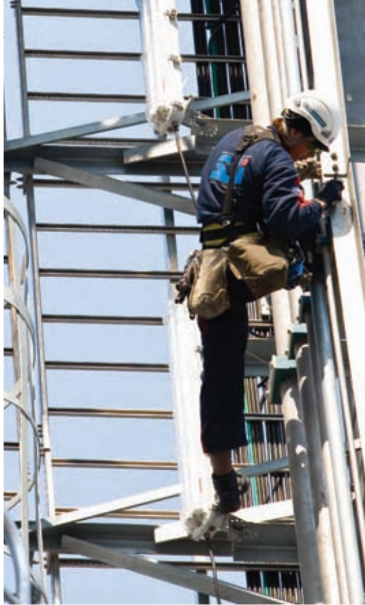
Pictured on page 38: Lance Netherland, Mechanical Supervisor I
