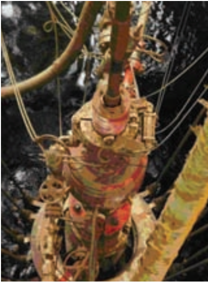
Transocean's concentric riser during drilling operations on board the Deepwater Frontier.
