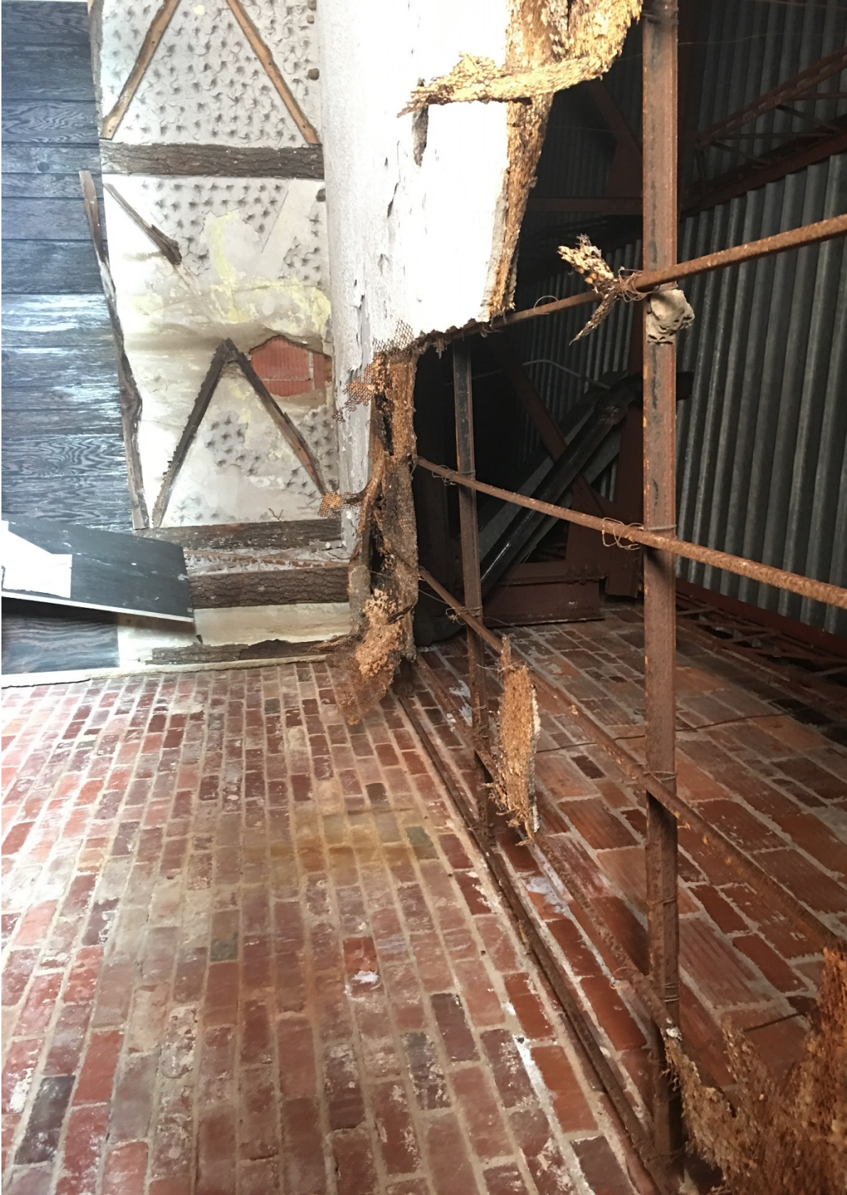
Deteriorated ceiling finishes and ceiling framing.
