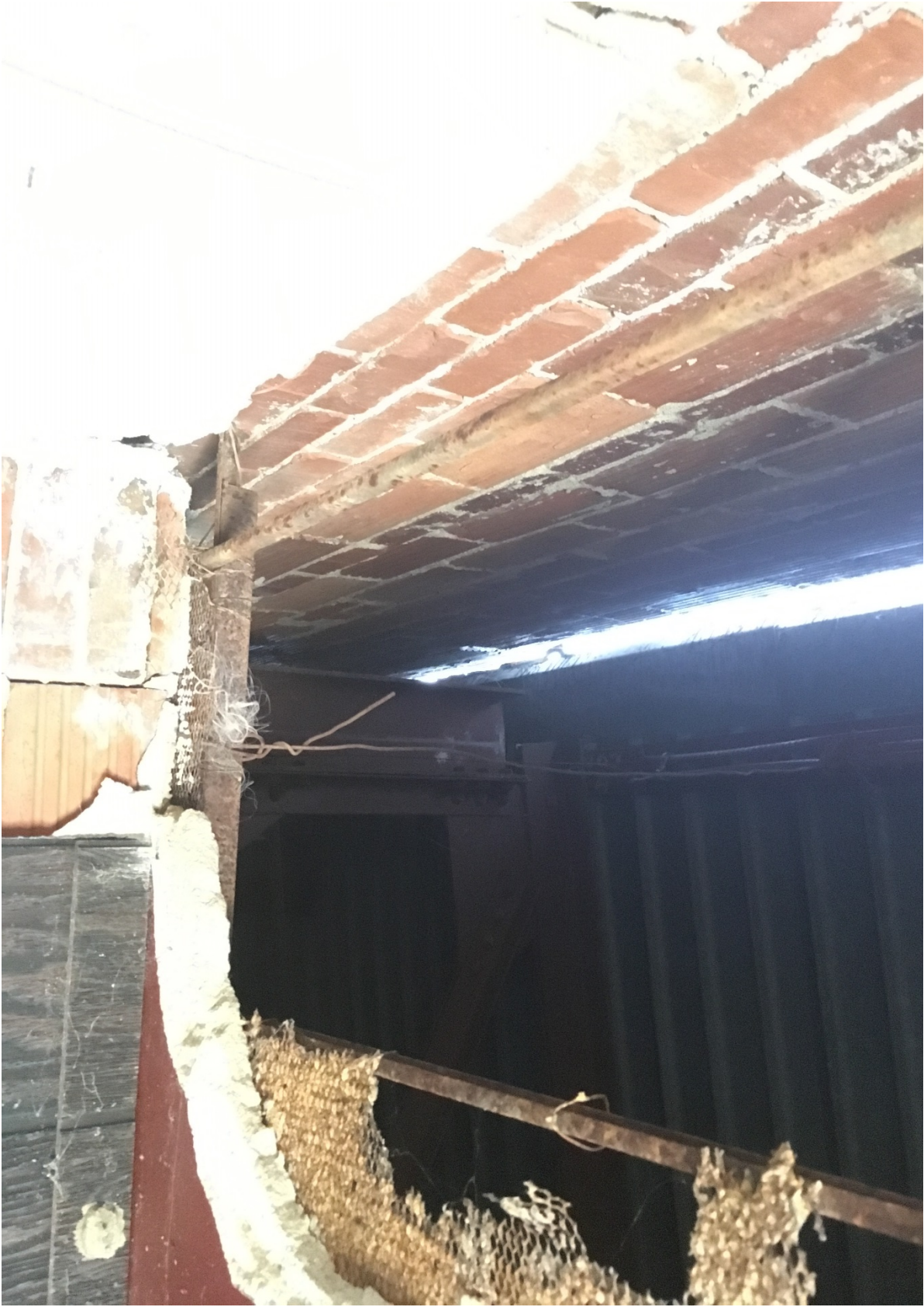
Gap at roof structure: South side of auditorium.
