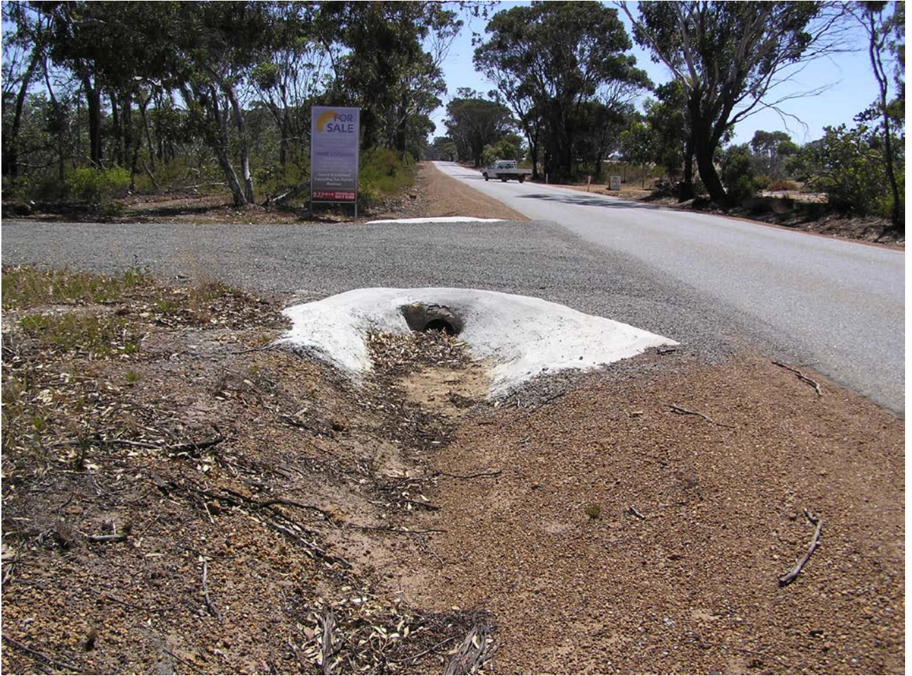
PLATE 5 - View to north along Albany – Lake Grace Rd looking showing existing driveway on western side of Albany – Lake Grace Rd and vegetation on verge which may need minimal clearing to allow for construction of the end taper for the proposed auxiliary right turn lane.
