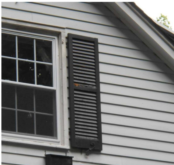
< The dirty look of this shutter is from the guano of bats roosting behind it. Also look for droppings beneath shutters.
