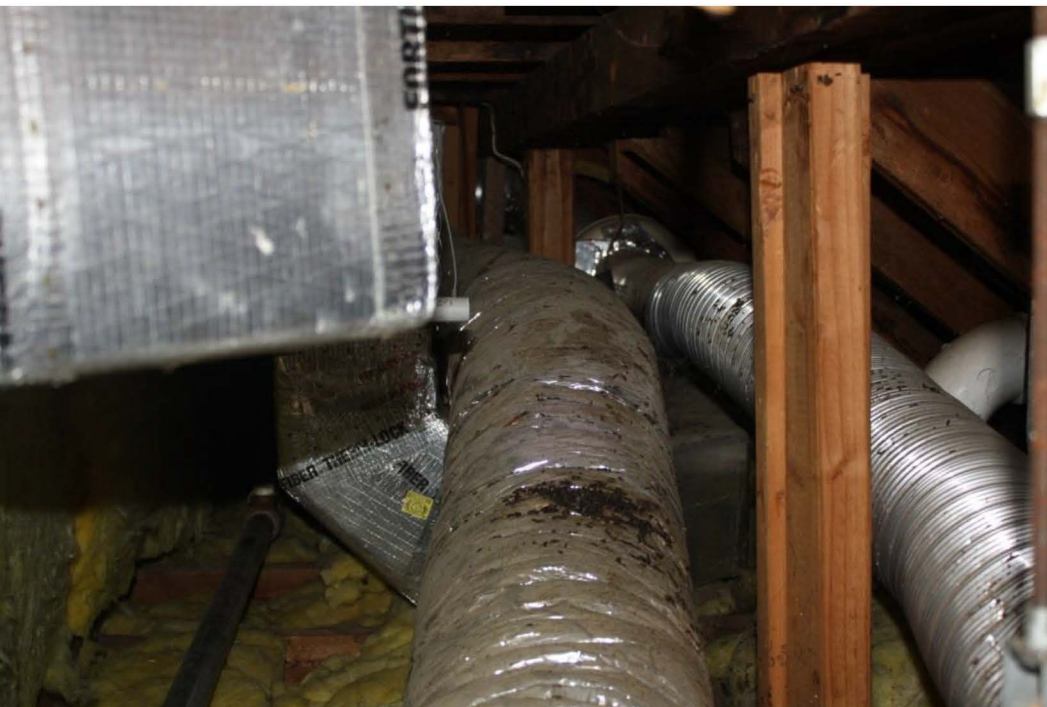
Small guano pile & some sprinkles on attic ducts
