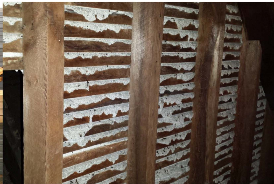
Guano visible on lath & plaster attic walls
