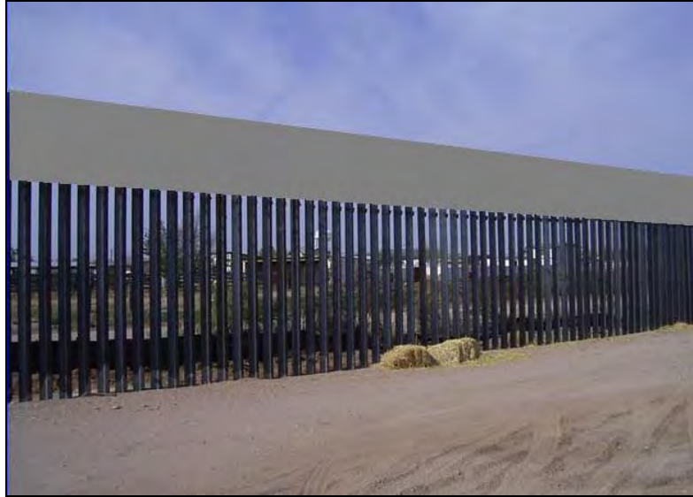
Figure 1-4. Personnel-Vehicle Fence Type-1 (PV-1)
