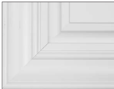
Example of front joint separation
