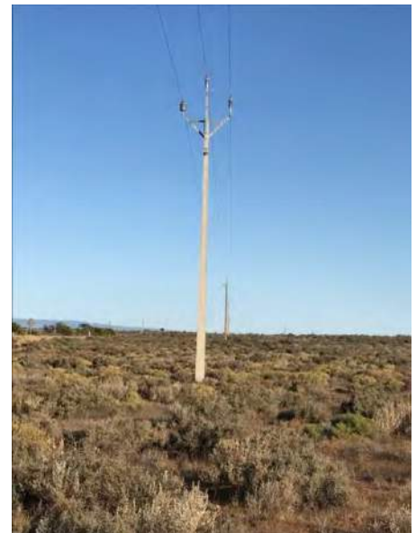
Figure 15 Example of a medium voltage power transmission line within the region.
