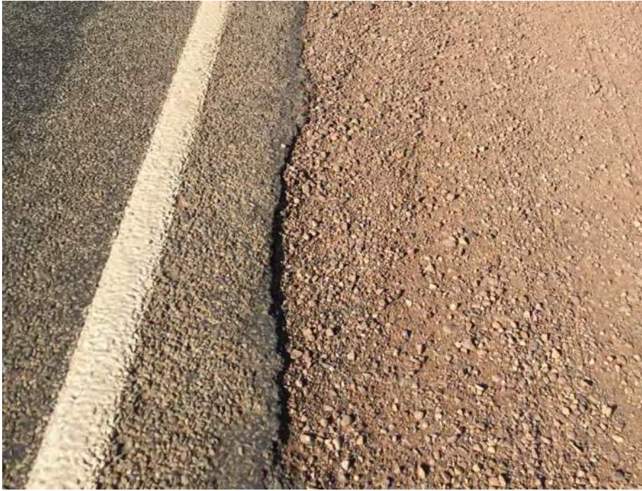
Figure 9 Minor edgebreak at proposed site access point
