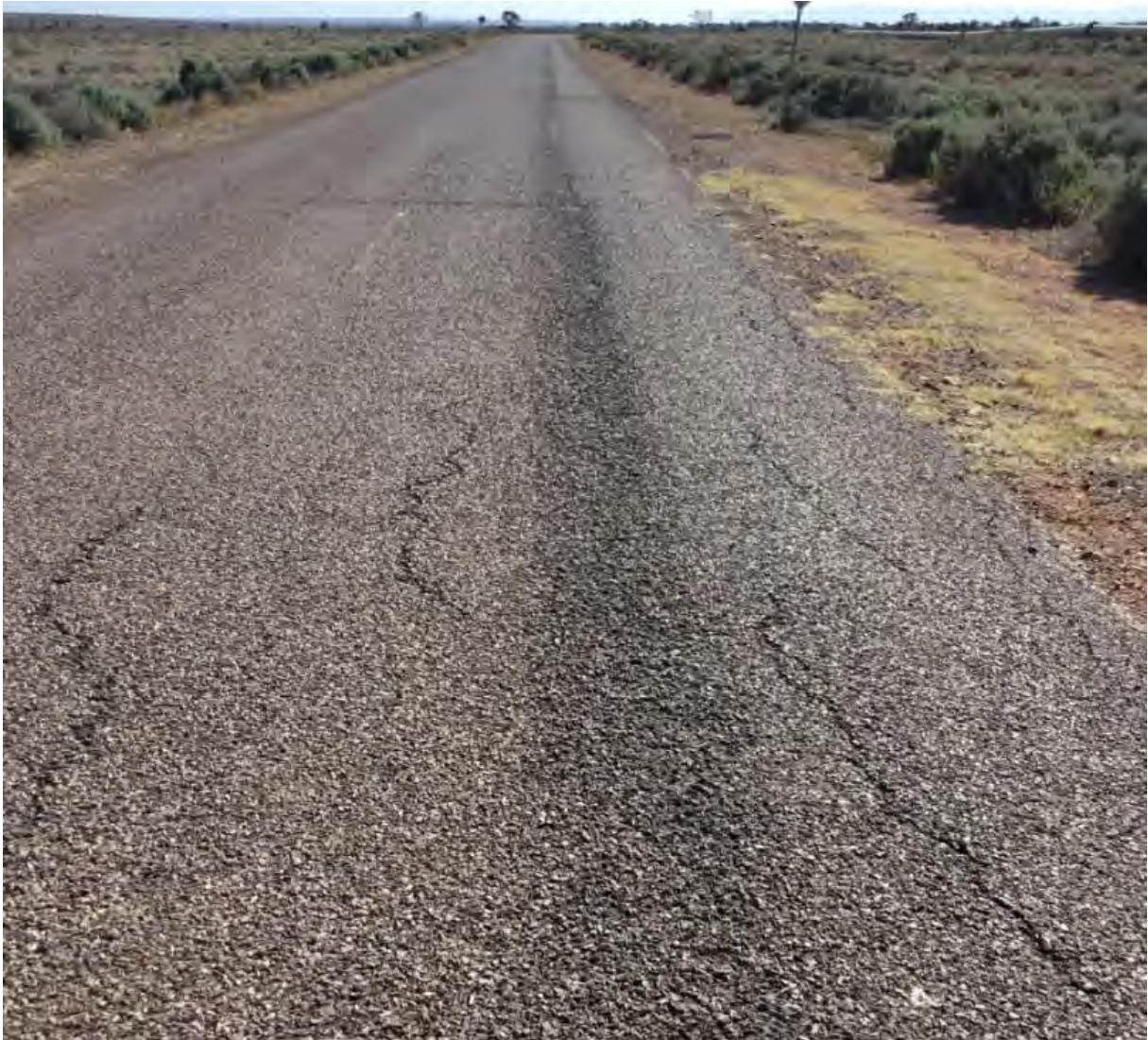
Figure 18 Longitudinal cracking on Caroon Road
