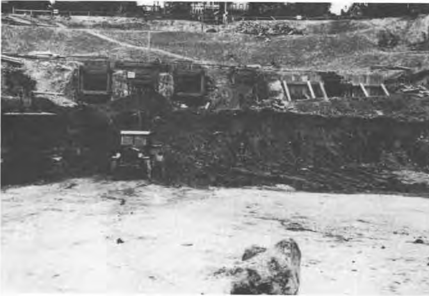
West portal drift excavations for tunnels through Mt. Baker Ridge, Seattle. These two double-lane tunnels were driven by the stacked drift method through glacially over-ridden hard clay. Note the large glacier-transported boulder in the foreground. 1939 photograph courtesy of Shannon & Wilson, Inc.
