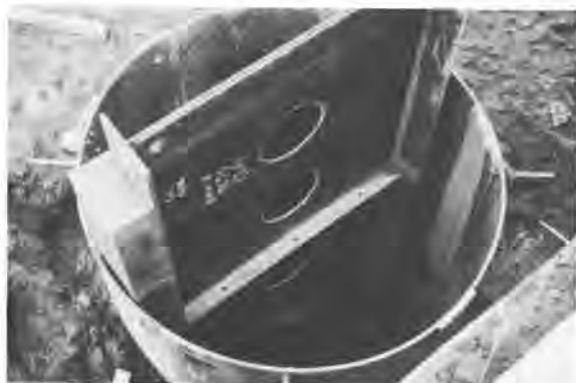
Figure 5. Cylinder pile (diameter 4 ft 9 in.) at the toe of an existing conventional wall. Steel beam is in place and ready for concrete pour.
