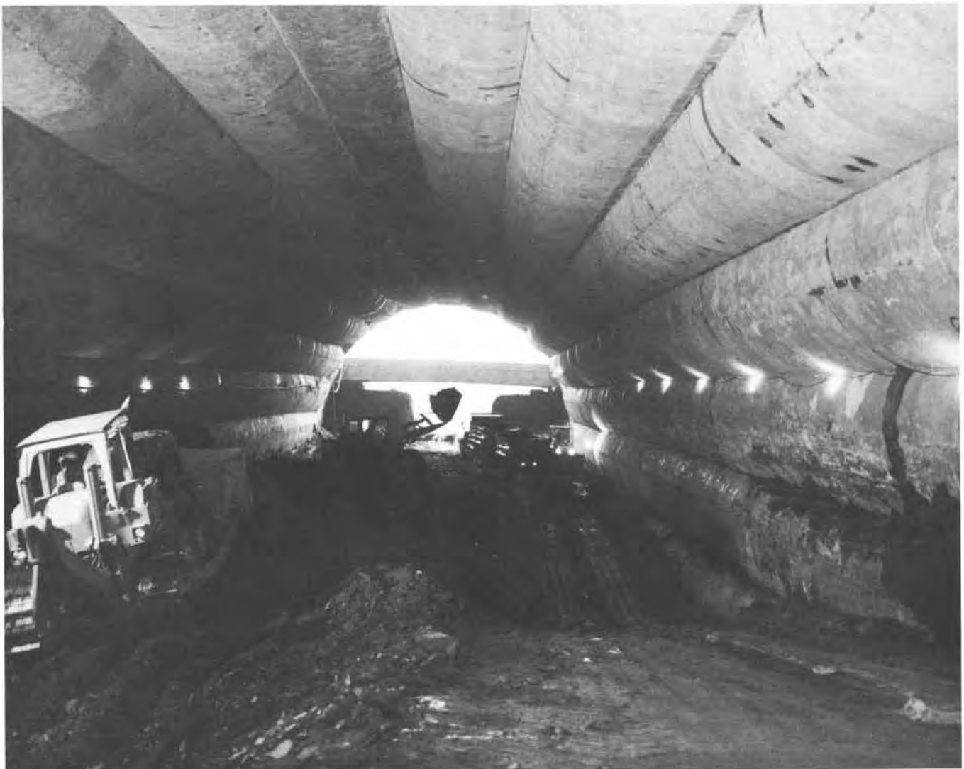
Figure 12. Excavation of bench #3 showing drift exterior and east access pit with upper level bracing.
