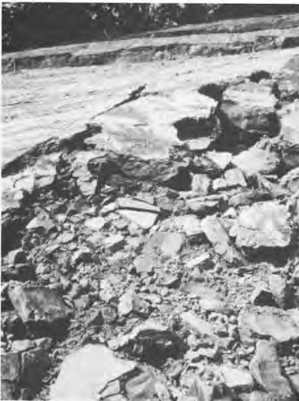
Figure 2. Hard blocks and chunks of clay in a landslide mass. Largest chunk in the upper middle part of the photograph is about 5 ft across.
