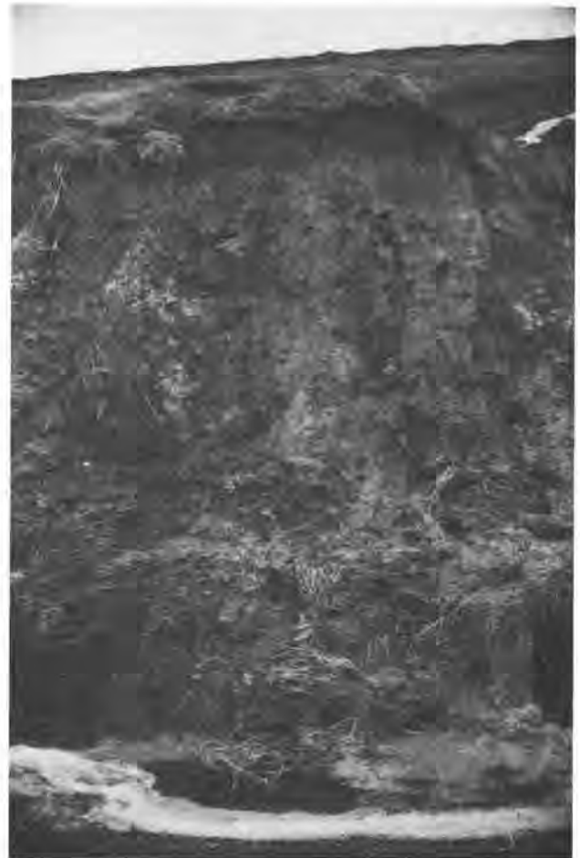
Figure 16. Small flow of soil and vegetation in a 15-ft-high cut slope along U.S. Highway 195 near Pullman.
