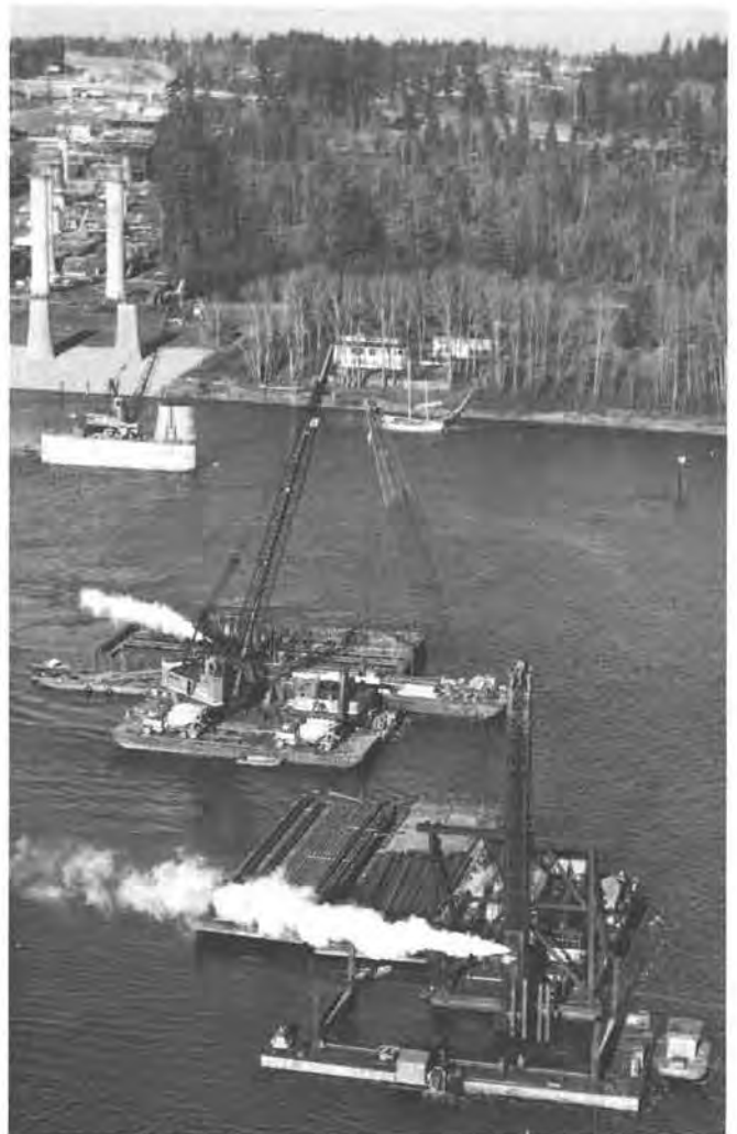
Pile driving for bridge piers at the Glenn Jackson Bridge site, 1978. Photograph courtesy of the Oregon Department of Transportation.
