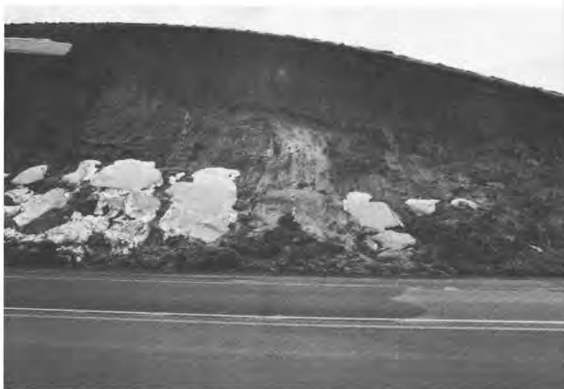
Figure 17. Failure of cut slope in clayey loess near Pullman. White areas are snow. Cut is about 30 ft high.
