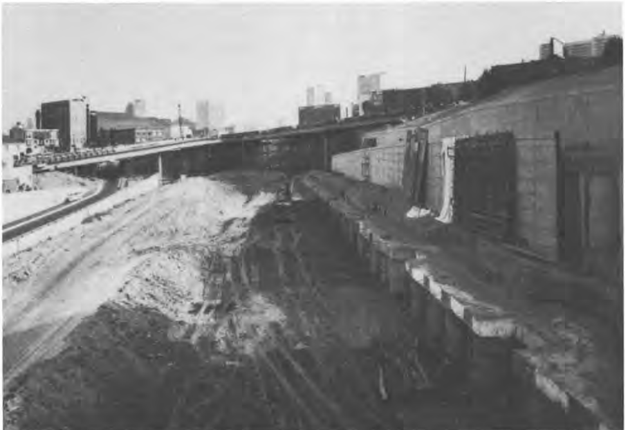
Figure 10. View north along the southbound lanes at the intersection of Boren Street and Pine Street. Two cylinder pile walls (10-ft diameter) were designed to accommodate the reversible lane under the southbound lane.
