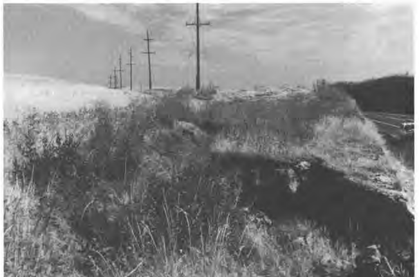
Figure 13. Gully erosion in a side ditch due to insufficient channel protection (U.S. Highway 12 near Walla Walla).
