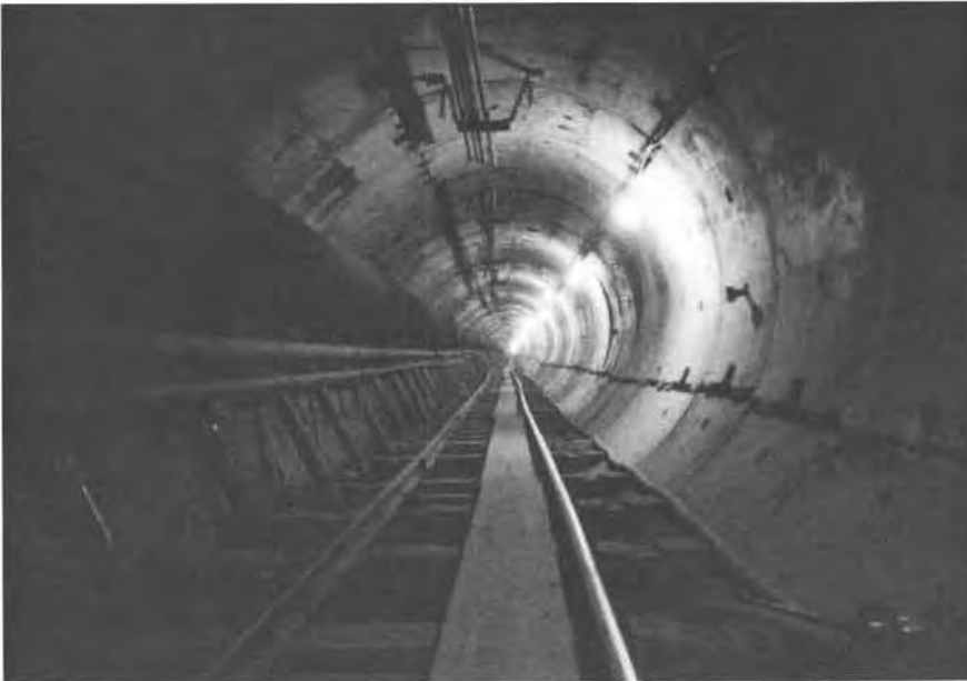
Figure 11. Temporary 5-in.-thick concrete segment lining for drift #3 with exterior lining of prior drift #1 on the left, wood wedges for liner expansion on the right, and grout lines in the crown.
