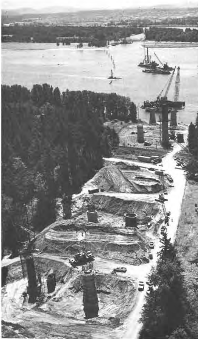
Bridge pier construction on the north (Washington) shore of the Columbia River, Glenn Jackson Bridge site in July 1987. Photograph courtesy of the Oregon Department of Transportation.
