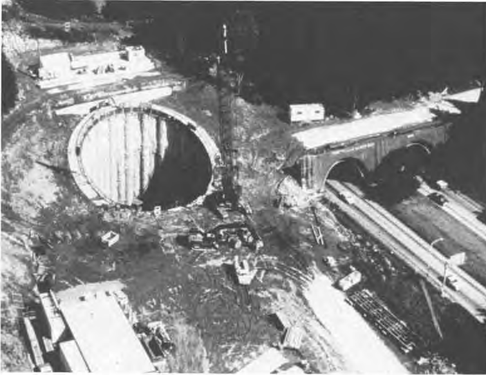
Figure 9. Aerial view of completed west access pit; existing tunnels on the right, stabilizing blocks above portal, construction yard to bottom.
