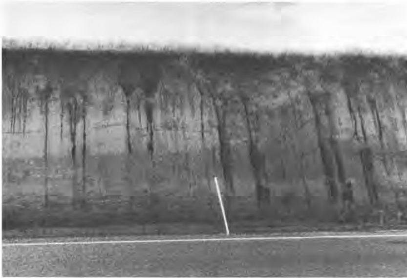
Figure 14. Erosion pipes developing into gullies on a 30-ft-high cut along U.S. Highway 12 near Walla Walla.
