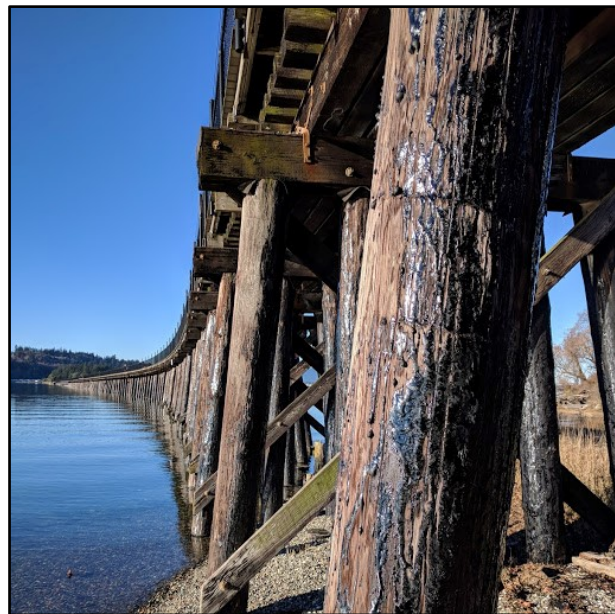
Figure 13. Creosote pilings support the Tommy Thompson recreational trail across the bay. View looking west. (DNR Photo)
