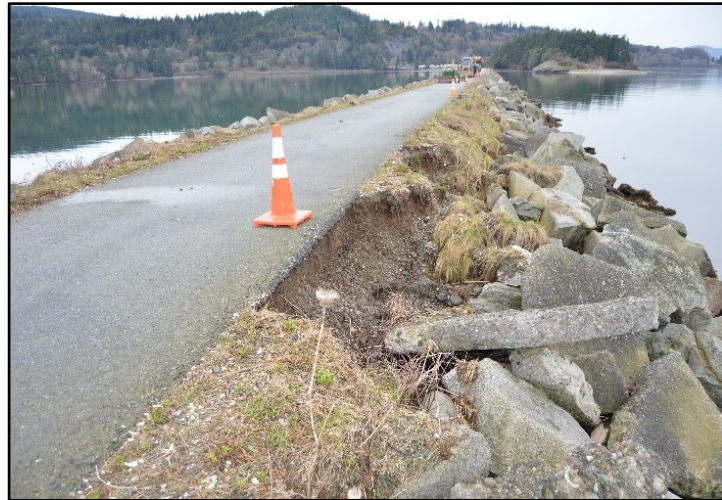
Figure 15. Damage to the causeway revetment from storm surge (DNR photo)
