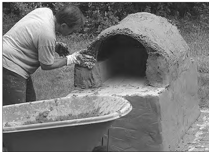
The wood-fired pizza oven under construction. Ronald Hirsch applies the adobe clay around the door area. AP Photo
