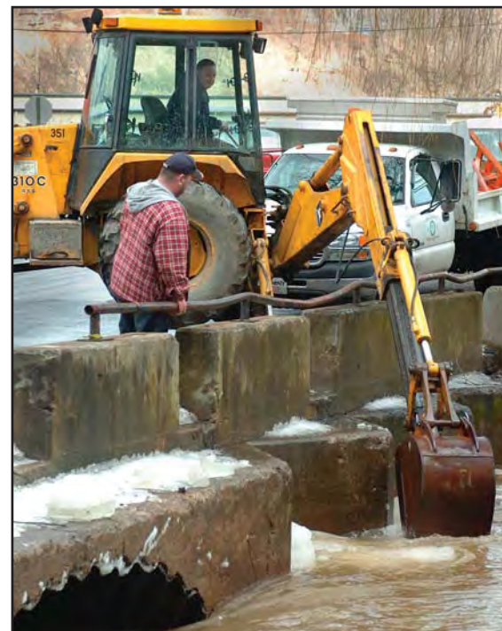
Public Works crewman John Schumber (front) watches as coworker Rod Squires dislodges the ice jam with an excavator blade on a backhoe.
