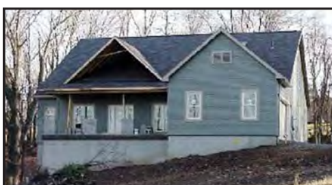
4 Hoot Owl Lane $435,000 Elegant living on one floor...less than 10 minutes from Morgantown is this new construction. Over 2400 sq. ft. of convenient living. This home features hardwood floors, fireplace, maple cabinetry and stainless appliances.
