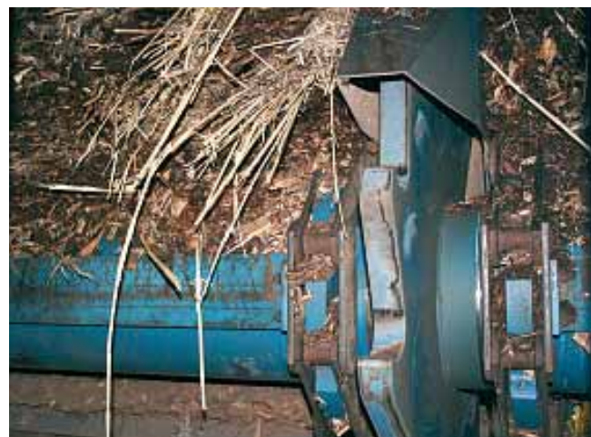
Reed going to a boiler together with woodchip in Perniö, Finland, in June 2007. Long pieces of reed are not a problem in large-scale power plants like this one, but they can get badly stuck in small-scale boilers. Photo: Eija Hagelberg.
