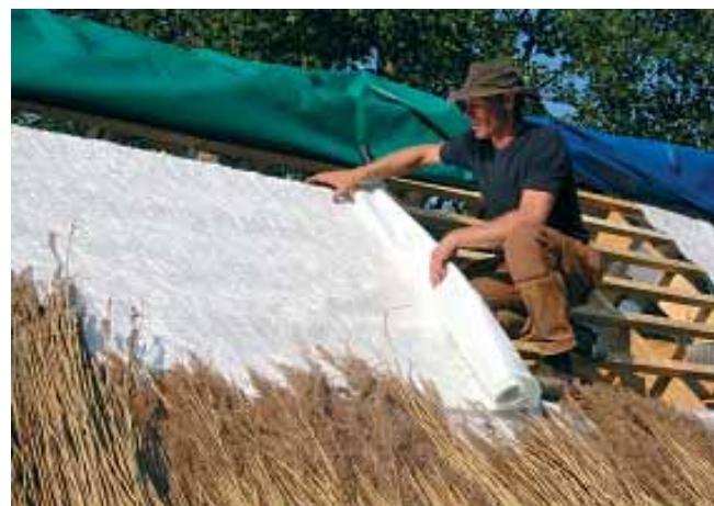
A fireproof fabric is laid out above the timber and below the reed. Photo: Carlo F. Christensen.
