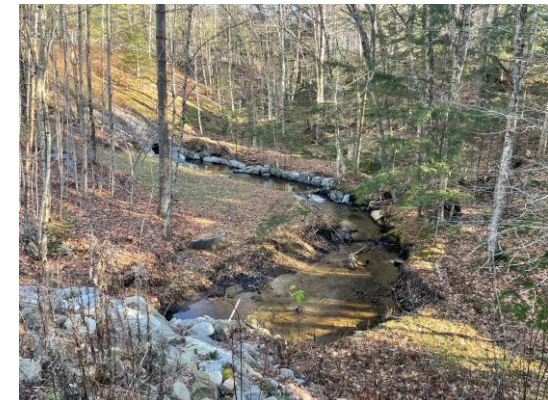
L: Route 28 over Unnamed Creek at Cliffhouse Road - showing perch and eroding bank.
