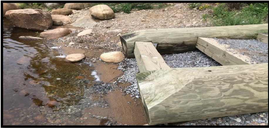
Picture from 2021 showing erosion of bottom step from high water events along the Moose River.
