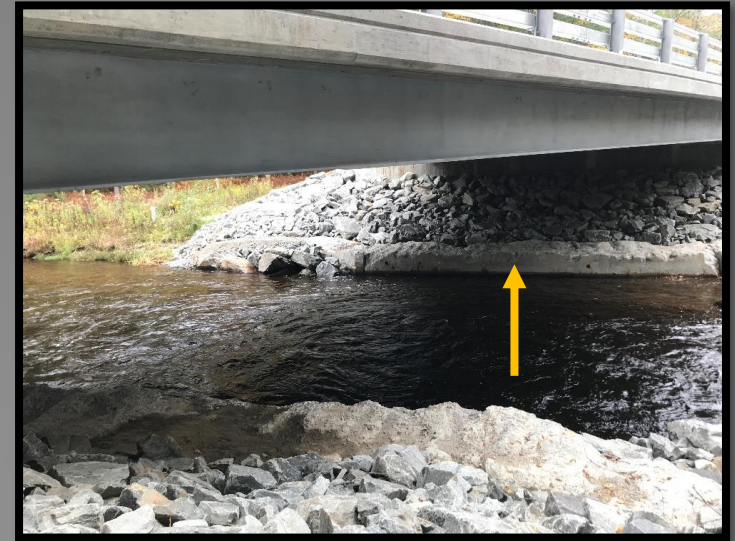
The portion of terrestrial trail under the bridge incorporated the partially demolished former concrete bridge abutment.
