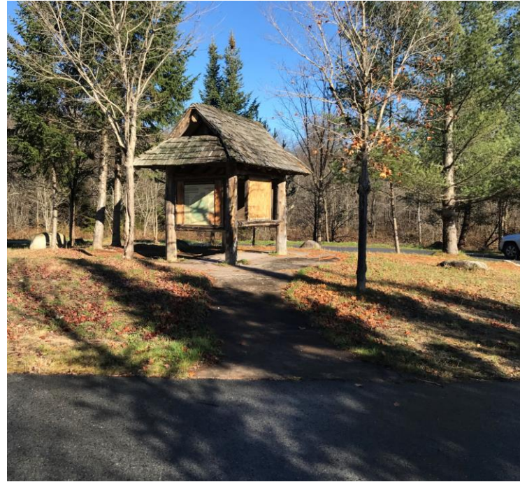
Kiosk on site with missing interpretive panel.
