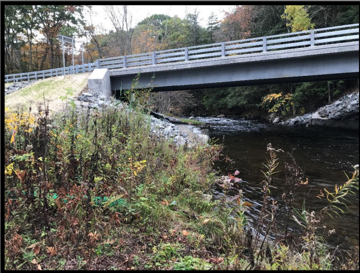
East End Abutment- topography too steep and unsuitable to install a terrestrial crossing
