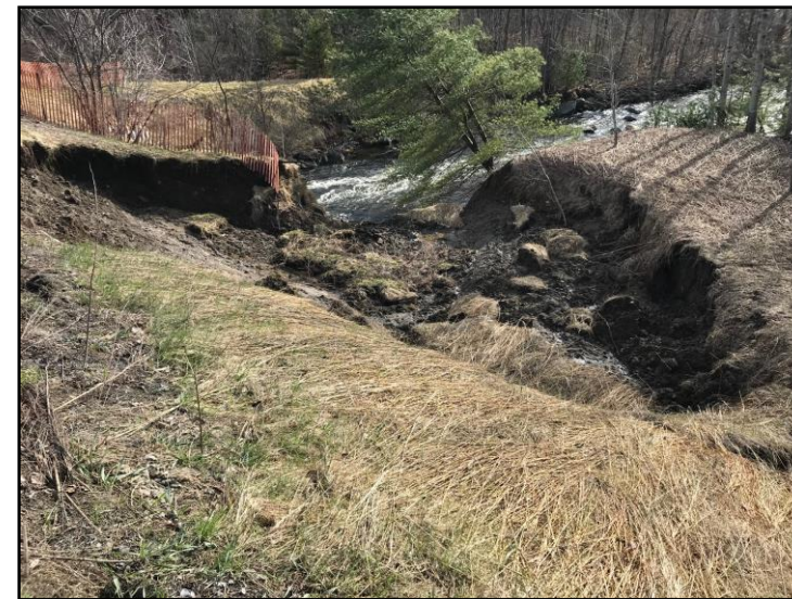
Fall 2018 slope failure
