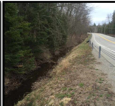
Saturated ditchline with standing water against highway embankment.
