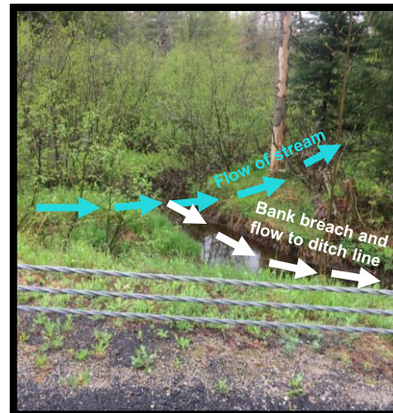
Existing streambank breach location in relation to road. Note abundant alder shrubs.
