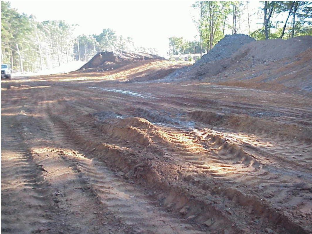
Figure 31 Haul Road Damage
