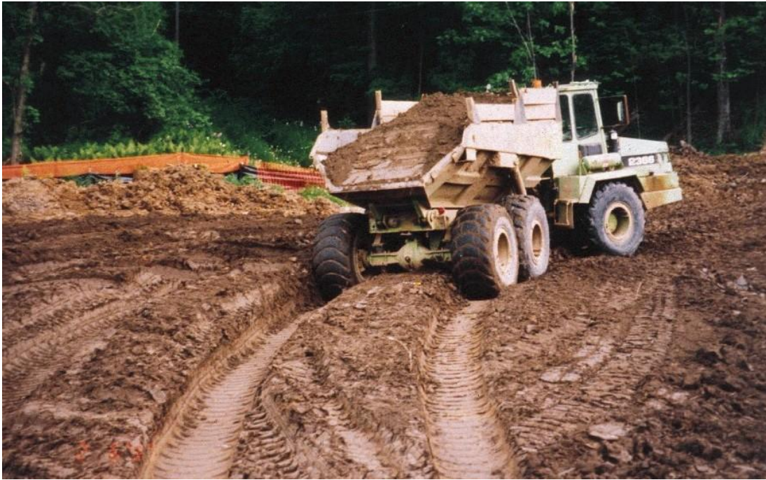
Figure 30 Haul Road Damage
