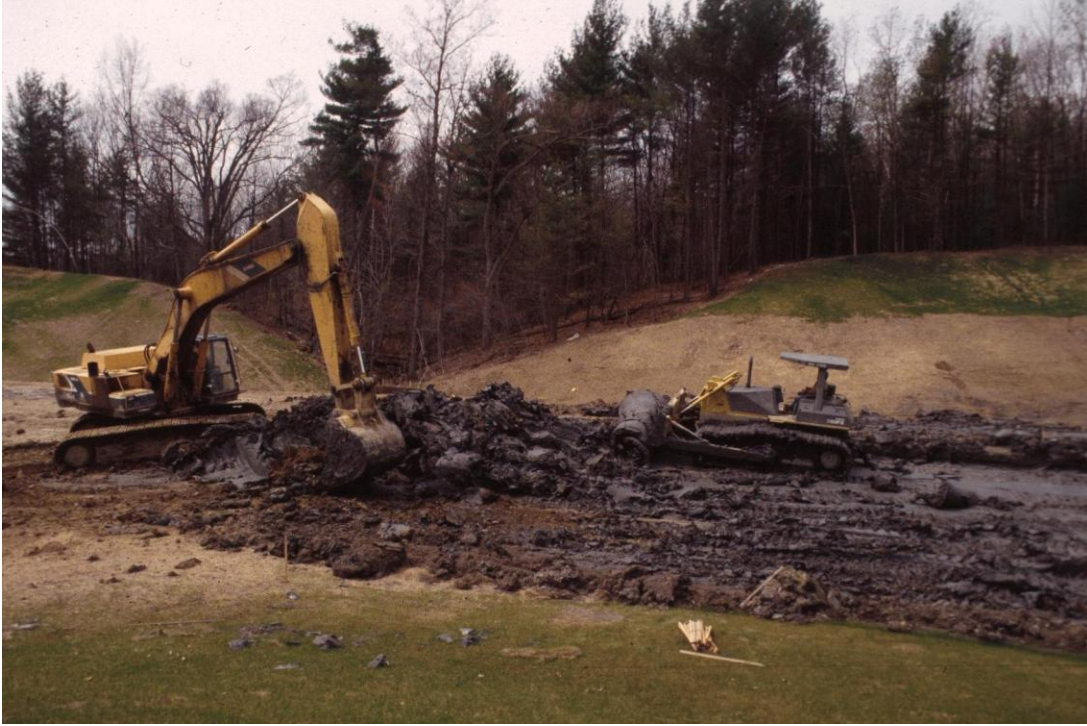
Figure 20 Unstable Embankment Foundation
