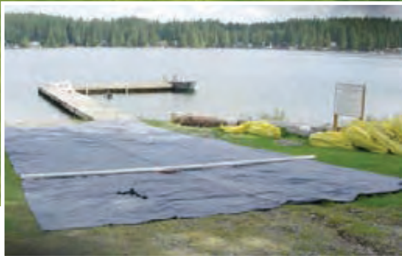
A geo-textile benthic blanket ready for installation in a Pacific Northwest Lake in the United States
