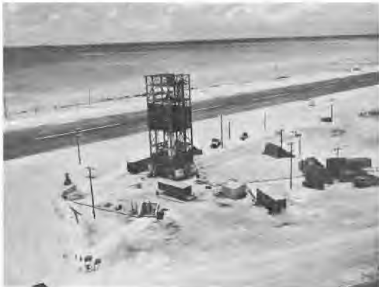
Figure 79. Launch complex at Johnston Island; HARDTACK, TEAK Redstone is in the gantry.
