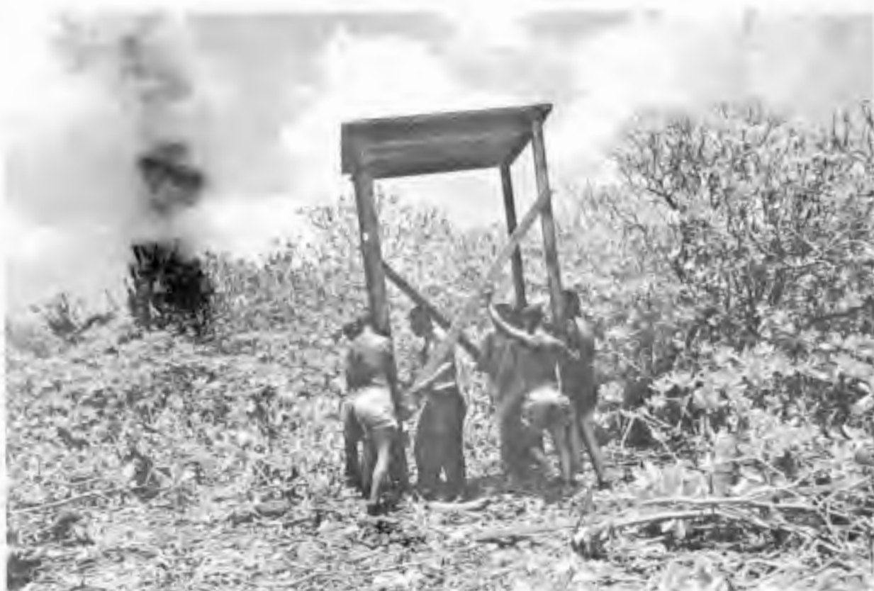
Figure 8. Small photo tower being built on Mut Island, Enewetak Atoll, in heavily vegetated area, 1958.
