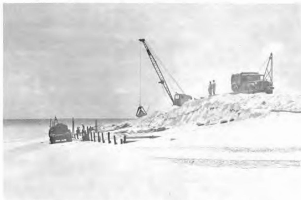
Figure 12. Revetment being built at west end of Eneman Island, Bikini Atoll (tip of ZUNI crater), 1958.
