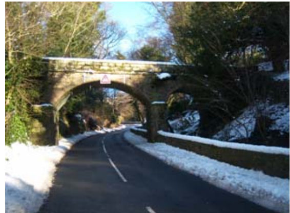
Looking up the B6281 towards the footbridge over the road and the Hell Beck
