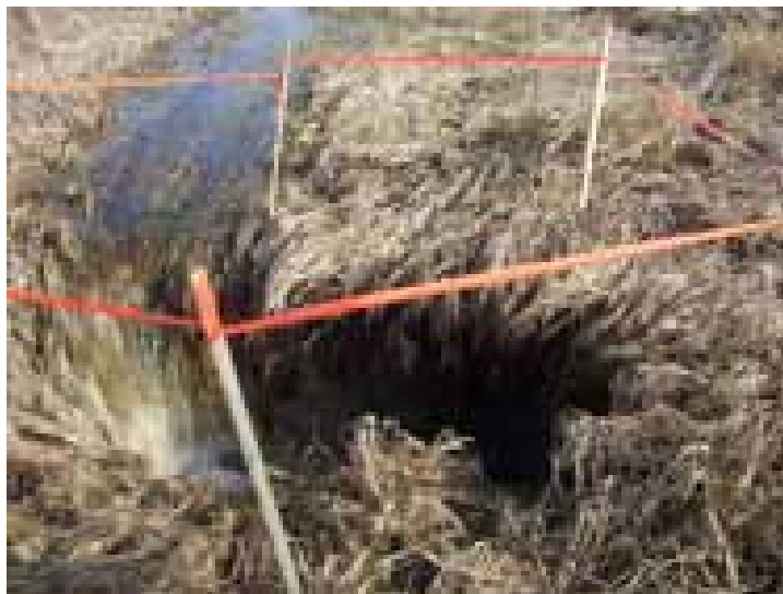
Figure 20: Sinkhole in the Grassmere Drain (2008)
