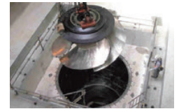
Drainage pump facility
