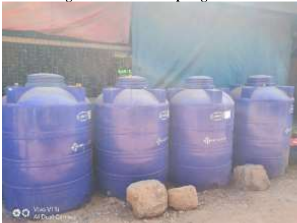
Figure 5-37 Water Storage Tank
