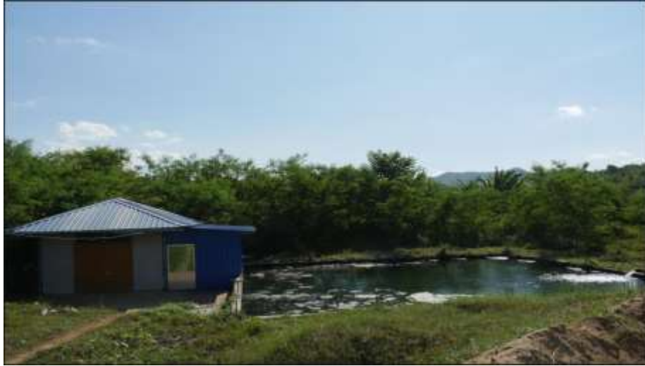
Figure – 44: Part of ground tank and pump house
