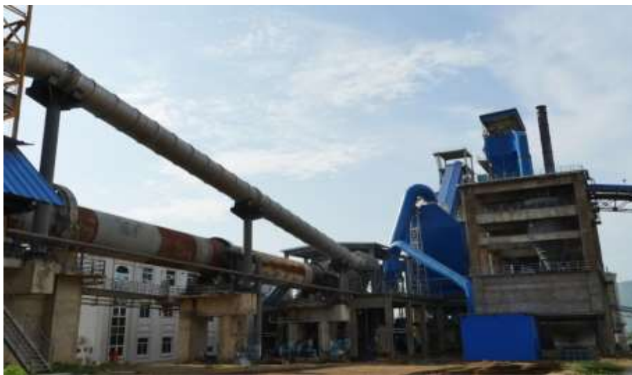
Figure – 28: Rotary kiln (Length 54 m, diameter 3.5 m)
