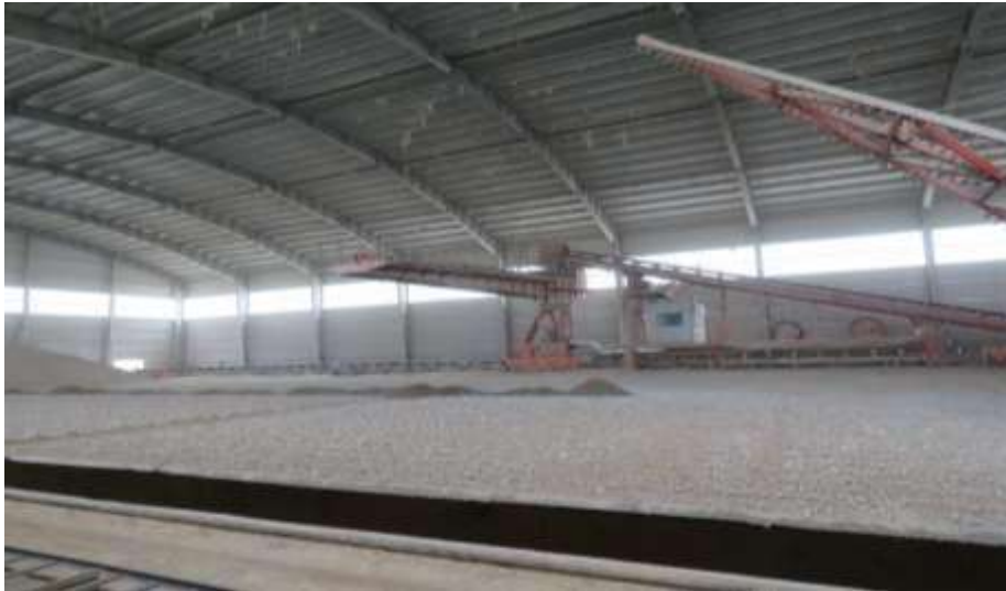
Figure – 21: Scraper reclaimer
