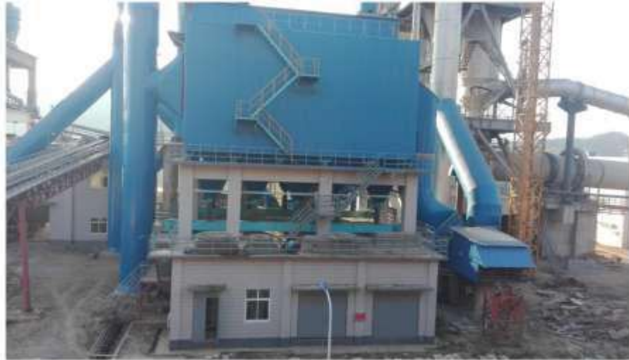
Figure – 100: Bag filter house
