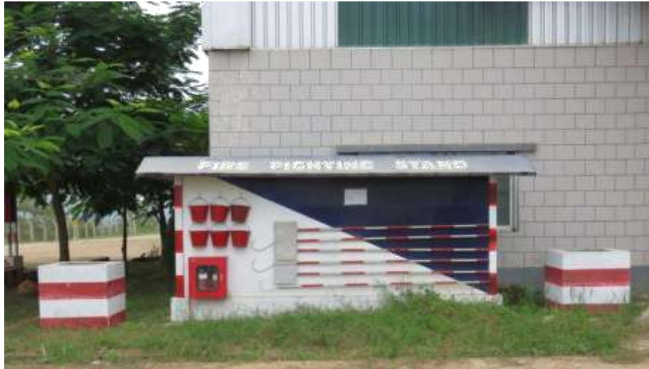
Figure – 115: Firefighting stands (traditional)
