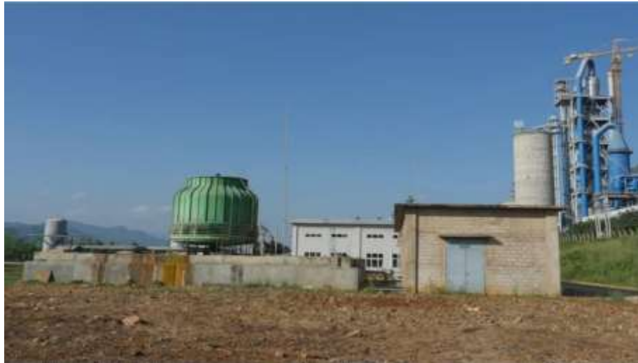
Figure – 105: Water treatment plant
