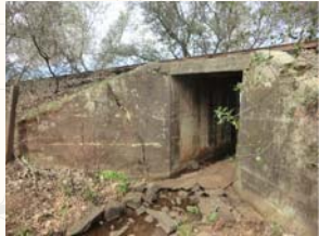
Location: MP 135.6 Crossing: Slate Creek Bridge Type: 60' open deck timber trestle with tamber piers and concrete abutments Condition: Poor. Timber piers need to be replaced
