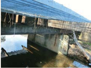
Location: MP 1278.63 Crossing: Little Indian Creek Bridge Type: 20' open deck timber trestle with steel stringers and walkways Condition: Good. Needs ties and approach work
