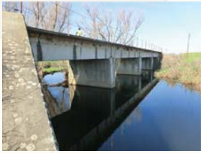
Location: MP 119.51 Crossing: Carson Creek Bridge Type: 128' ballast deck bridge with concrete girders Condition: Very good, needs approach work and some ties
