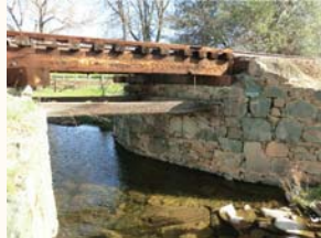
Location: MP 122.97 Crossing: Deer Creek Bridge Type: 12' open deck timber trestle with stone abutments Condition: Good. Needs ties, walkway, and approach work
