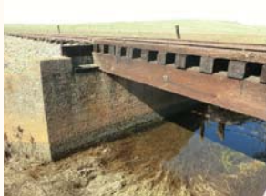
Location: MP 121.87 Crossing: Deer Creek Bridge Type: 15' open deck timber trestle without walkways Condition: Fair. Needs ties, walkway and one 8"x20" timber girder
