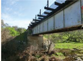
Location: MP 122.47 Crossing: Deer Creek Bridge Type: 68' ballast deck steel plate girder with walkways Condition: Good. Needs some ties and approach work
