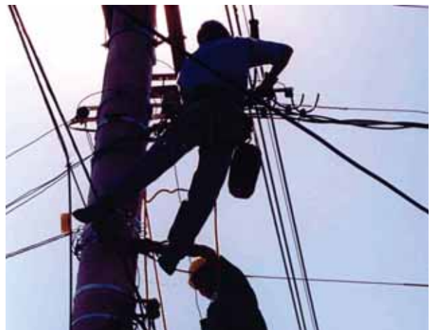
Grid maintenance Enersul
