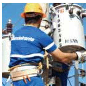
Grid maintenance Bandeirante
