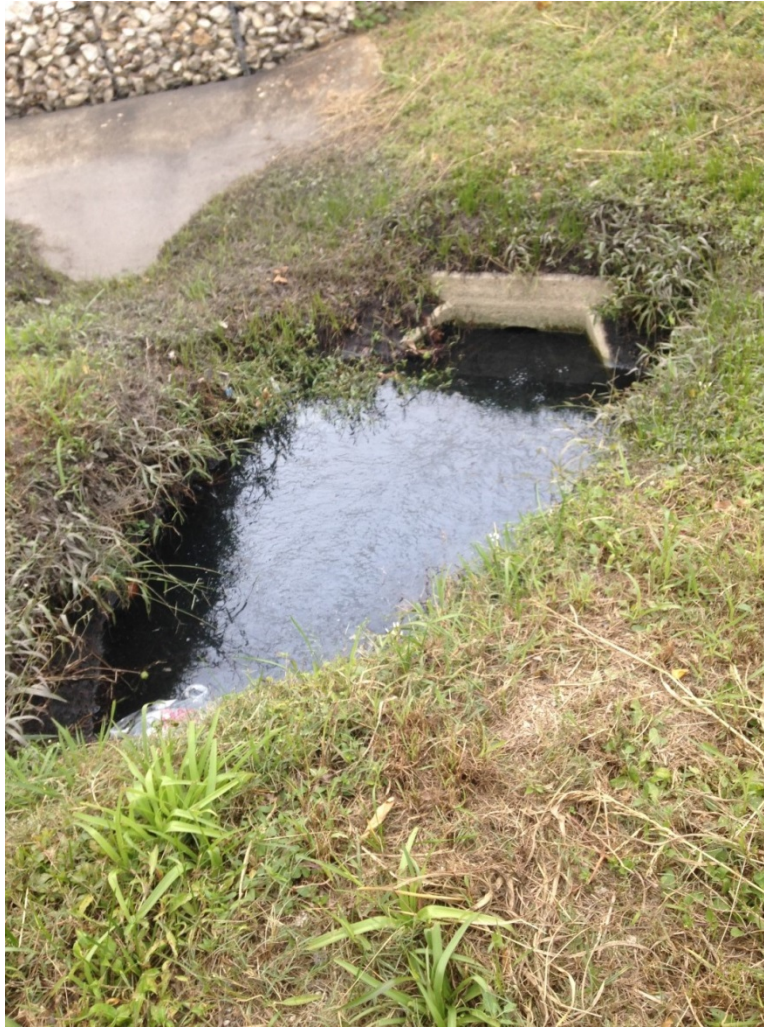
Figure 3-3 Third Storm Sewer Outfall Below Grade and Drainage Issue
