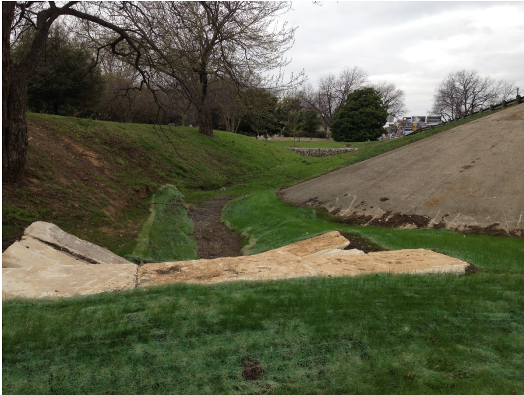
Figure 3-4 Erosion on Left Bank (Looking Upstream)
