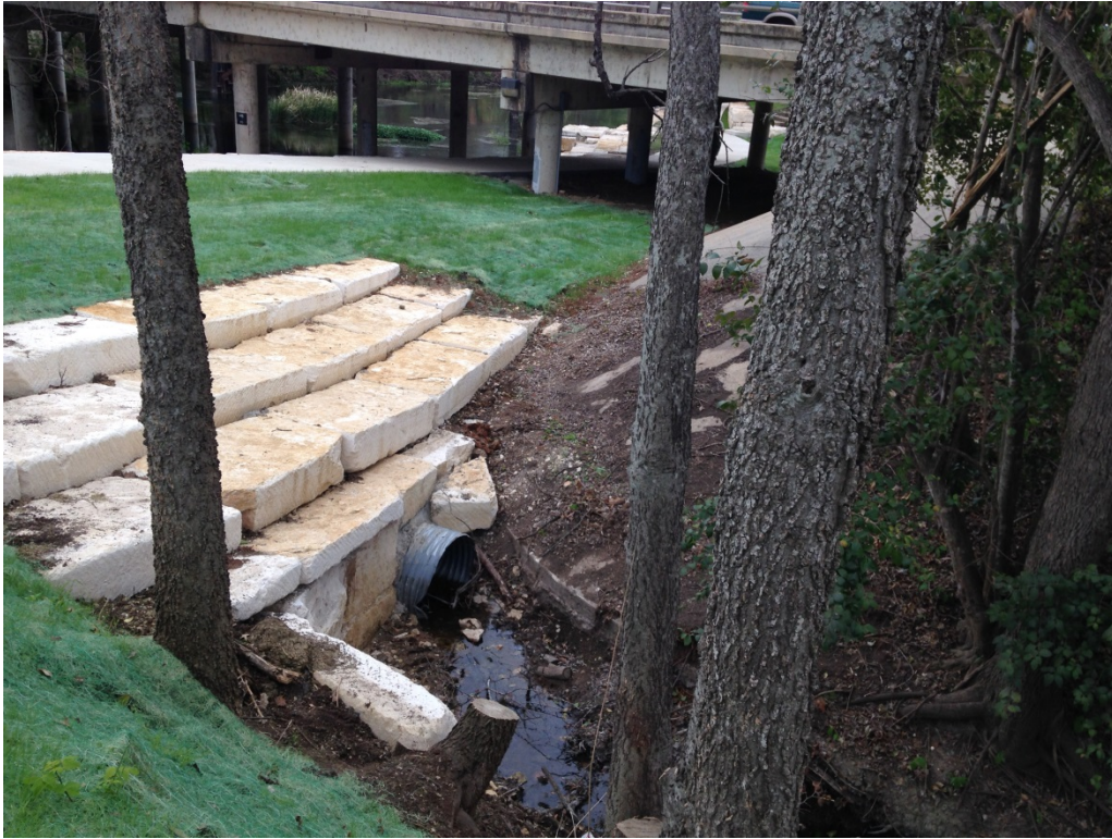
Figure 2-3 Existing Trail, Corrugated Metal Pipe Culvert, and Proximity to Bridge and River
