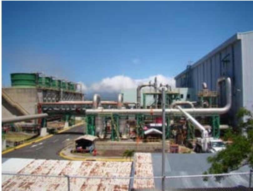
Photograph No. 1.2 of the distribution of the powerhouse and cooling tower constructions in Miravalles 1 - Photograph Rogelio Zeledón
