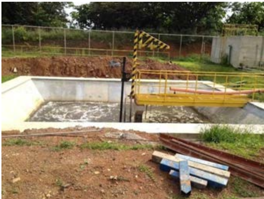
Photograph No. 5.18 Waste water treatment tank Pailas Geothermal Field Photograph Gabriela Zeledón
