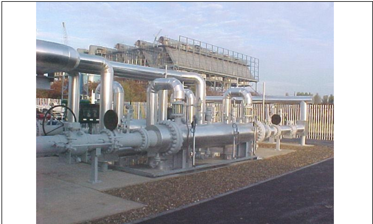
Fig. 1.2.6.-1 An Above Ground Installation site – interface point of the pipeline with the existing pipeline. The pipe is insulated
