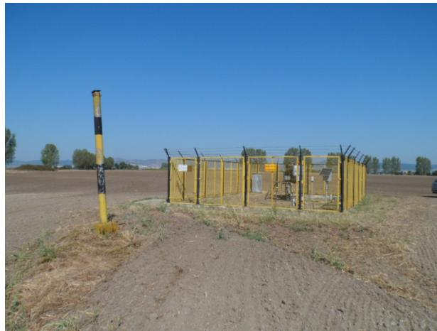
Fig. 1.2.1.7-2 – Existing AGI (Block Valve Station) at Stara Zagora
