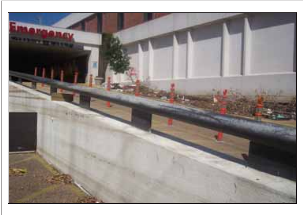
Figure 2-4. Damage at Lindy Boggs Center
