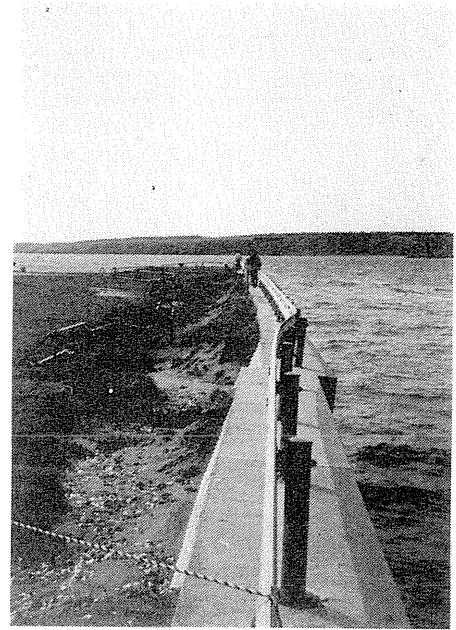
写真-5.2.5 花咲港地区B北側護岸のはらみ出し 中央部付近がはらみ出し、背後地盤が沈下した。 Photo-5.2.5 Large Movement of Quay Wall at East Pier The quay wall moved about 2 m and the ground behind the wall largely subsided due to liquefaction (Point B).
