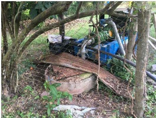
Groundwater well and pump
