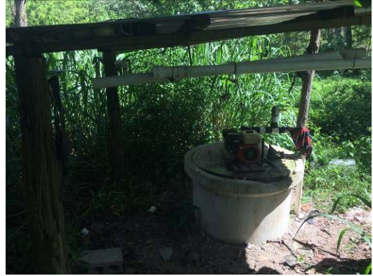
Groundwater well with pump in farm #108
