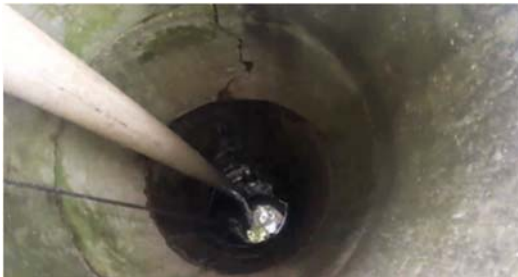
Underground well with pump beside Aguan River.
