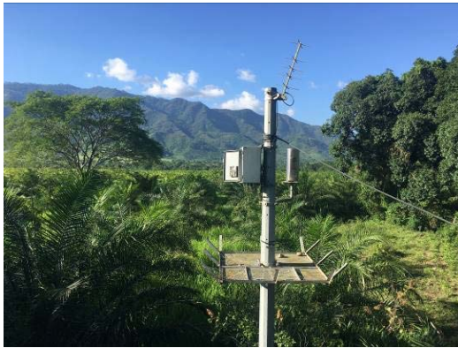
Abandoned/stolen meteorological station
