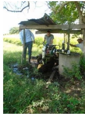
Underground well with pump beside Aguan River.
