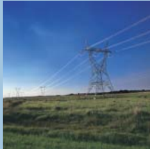
CIEI, Power Interconnection Argentina - Brazil
