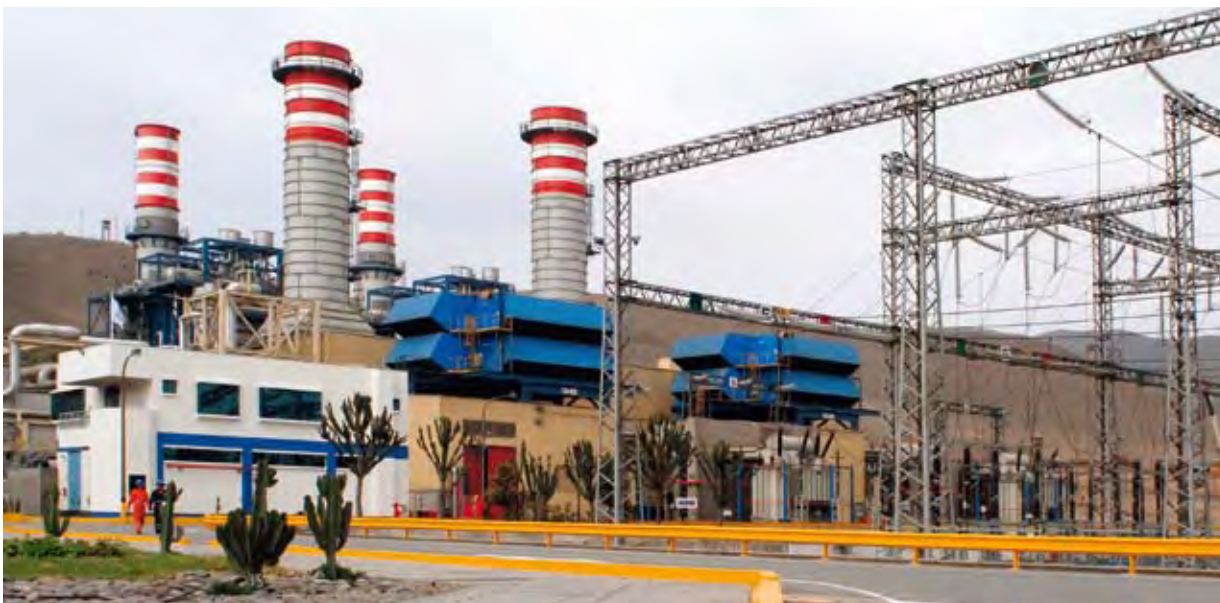
Power Plant Ventanilla, Peru
