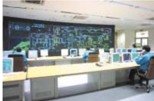
Load Dispatching & Control Center (Okayama)
