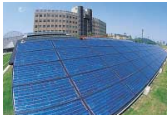
Photovoltaic power generation panel in the Technical Research Center
