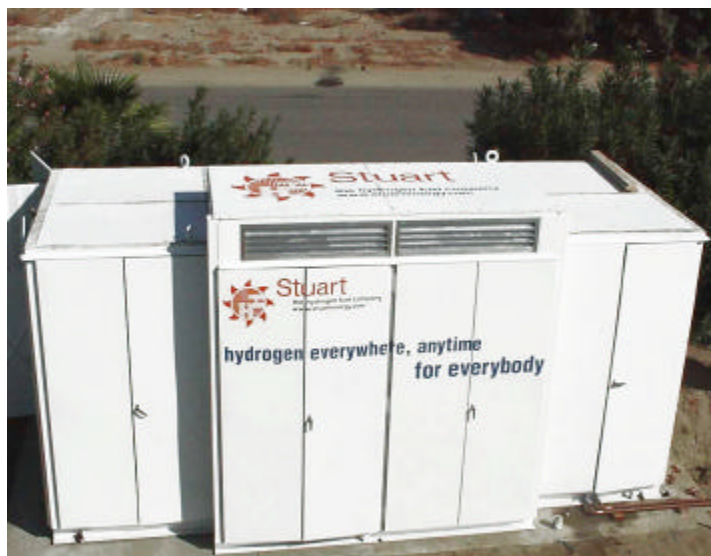
Figure 1 – The P3-1A Fleet Fuel Appliance at SunLine
