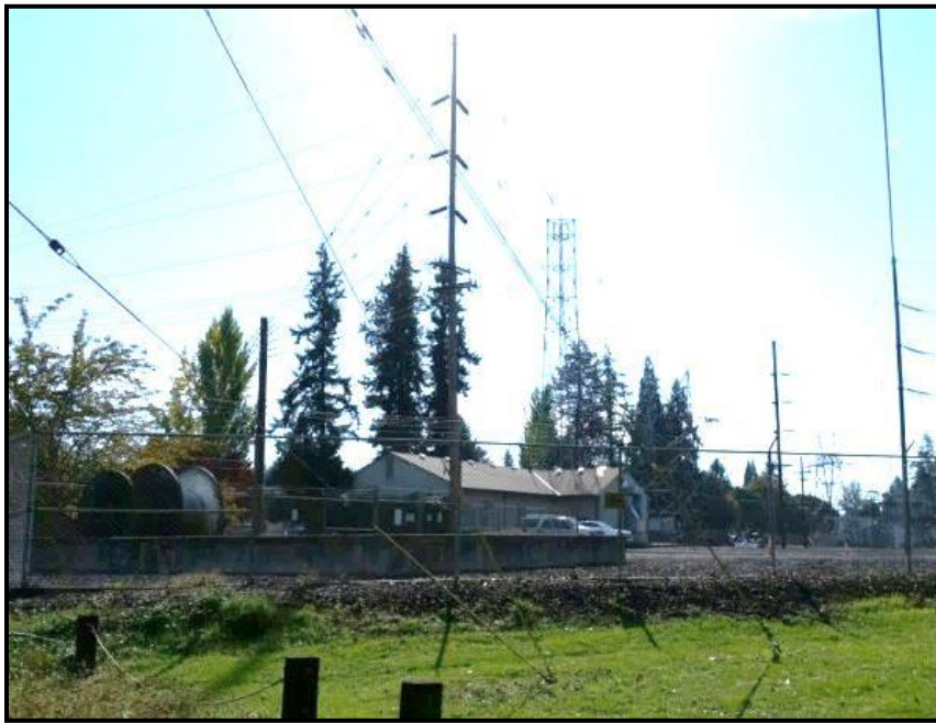
Photograph 2-11. BPA Albany Substation viewed from Hazelwood Park.
